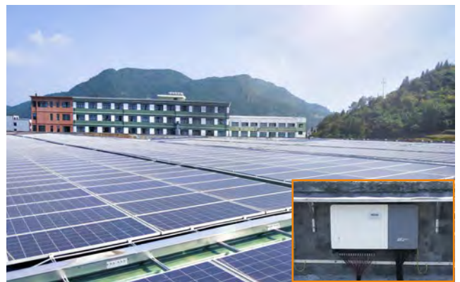
Tyco Electric, Panan Jinhua Zhejiang 1.5MW
