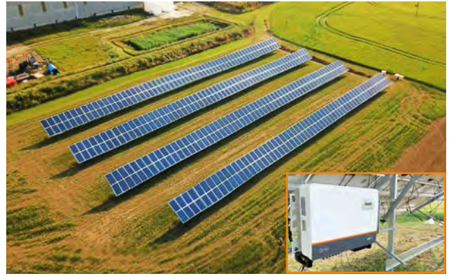
Lincolnshire, UK 140kW
