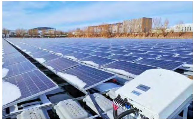
Beijing Shunzhen Green Harbor's Plant 5.5MW
