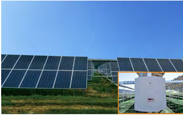
Hebei Zhangjiakou poverty alleviation PV Plant 5.1MW
