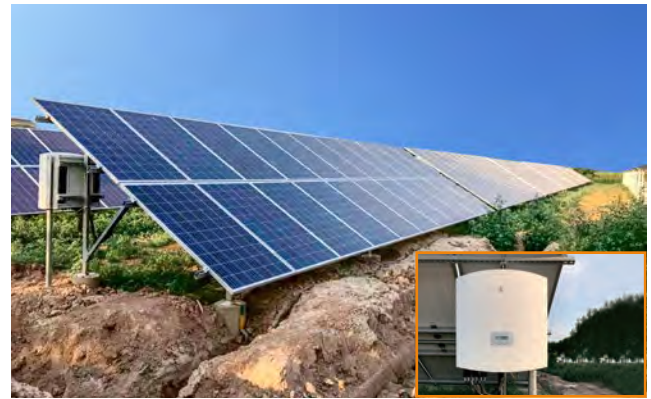
Hebei Qinghuangdao poverty alleviation PV Plant 5MW
