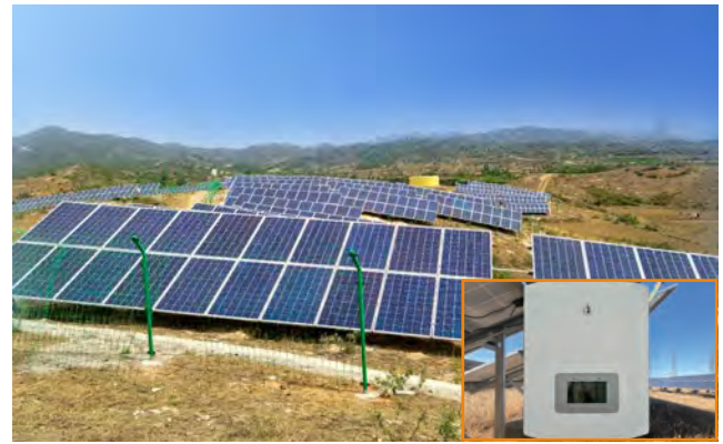
Hebei Qinghuangdao poverty alleviation PV Plant 9.7MW
