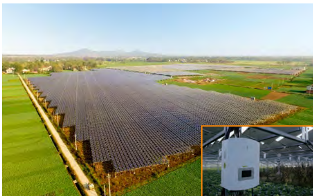
Hubei Guanyin Agricultural-photovoltaic hybrid PV plant 20MW
