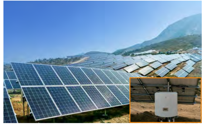
Liaoning Yingkou Jiuzhai PV plant 20MW
