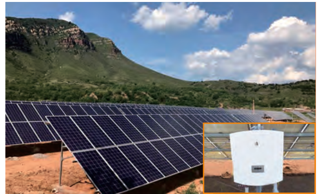
Shanxi Xiyang poverty alleviation PV Plant 7.2MW
