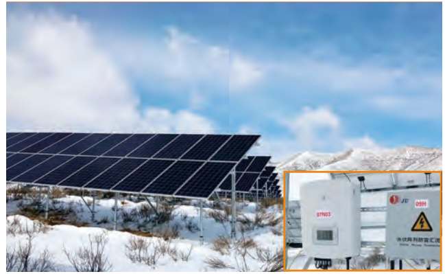
Shanxi Guangling PV plant 1.47MW
