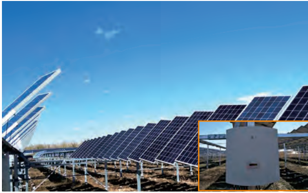
Hebei Zhangbei Agricultural-photovoltaic hybrid PV plant 50MW
