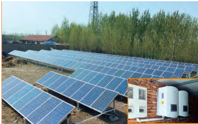
Shandong Leling poverty alleviation PV Plant 50kW
