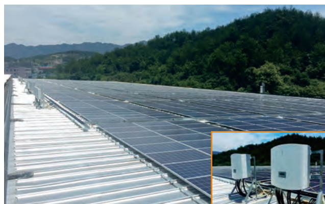
Hainan JiuLongGlass 1.7MW
