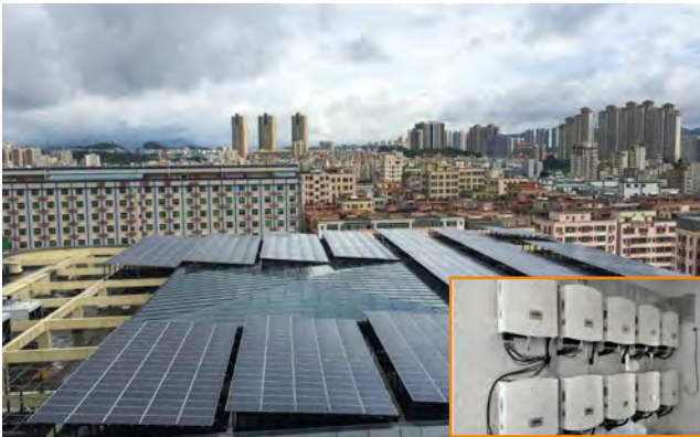
Shenzhen Jiangnan Times Building 600kW
